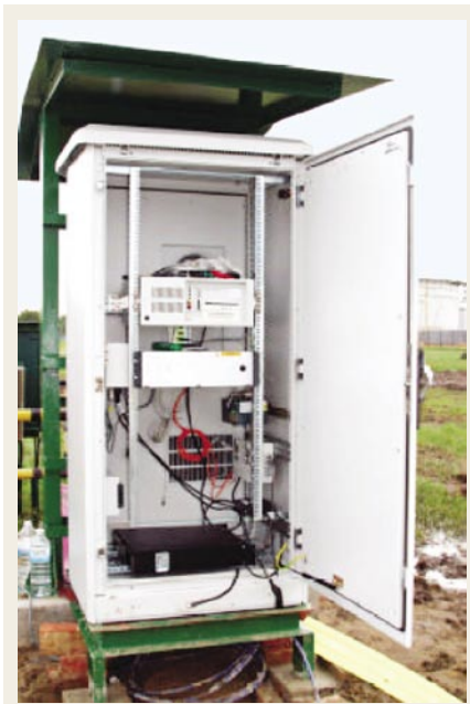
Fig. 2. Field cabinet with DTS (PC & OTS40P) equipment.
