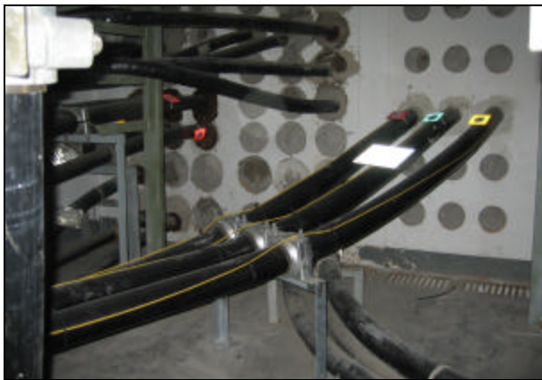
Fig. 1: Power cables with attached fibre-optic sensor cables (yellow)
