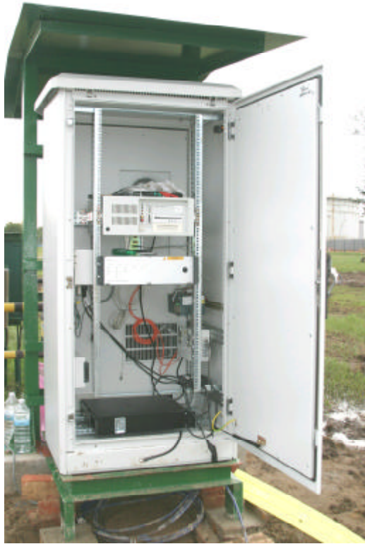
Figure 3: Field cabinet with DTS (PC & OTS40P) equipment
